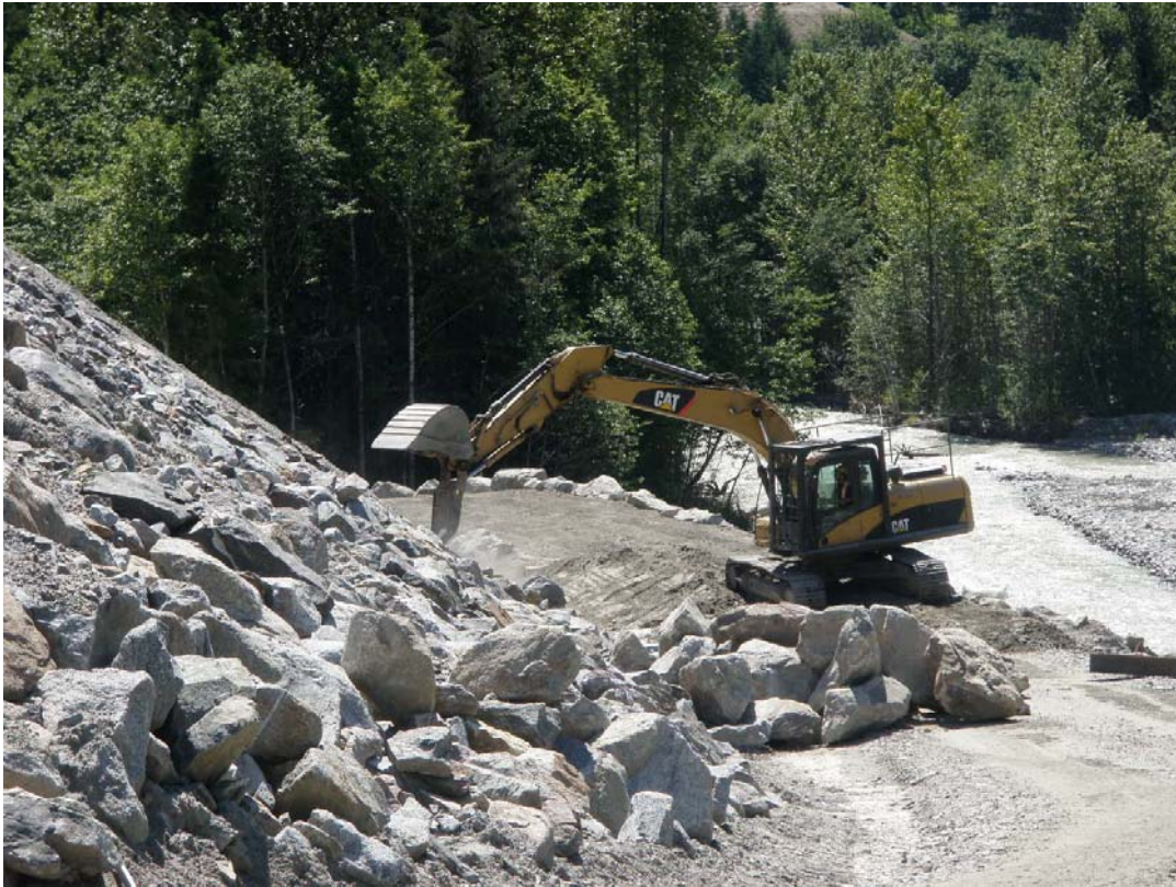
Sloping, ditching and placing armour along the East Toba tailrace access road. (July 10, 2010 12:02)
